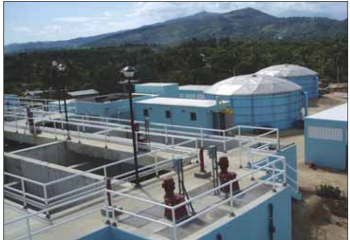
San Cristobal balance tank and chlorine contact tank.
