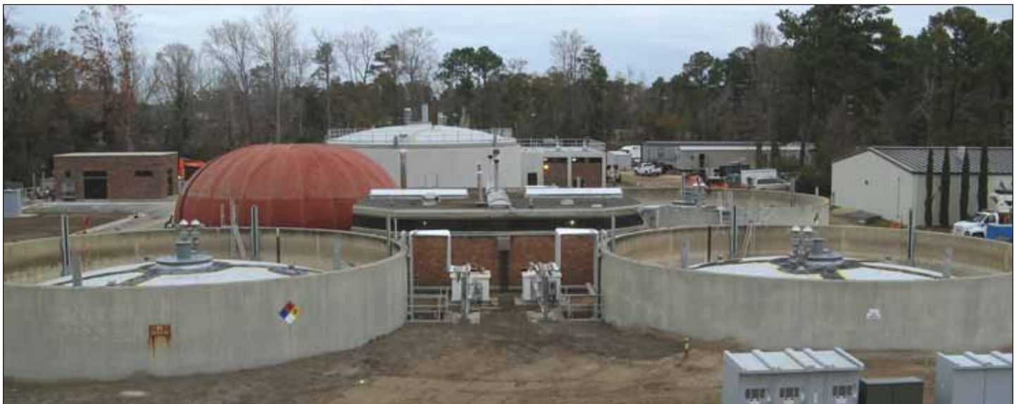
Digester gas storage is provided via gas holder style floating covers and ground level DYSTOR™ membrane gas storage.
