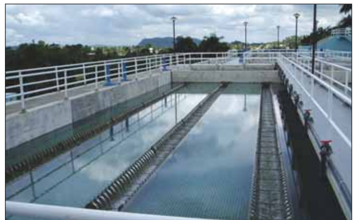
San Cristobal filter basin.
