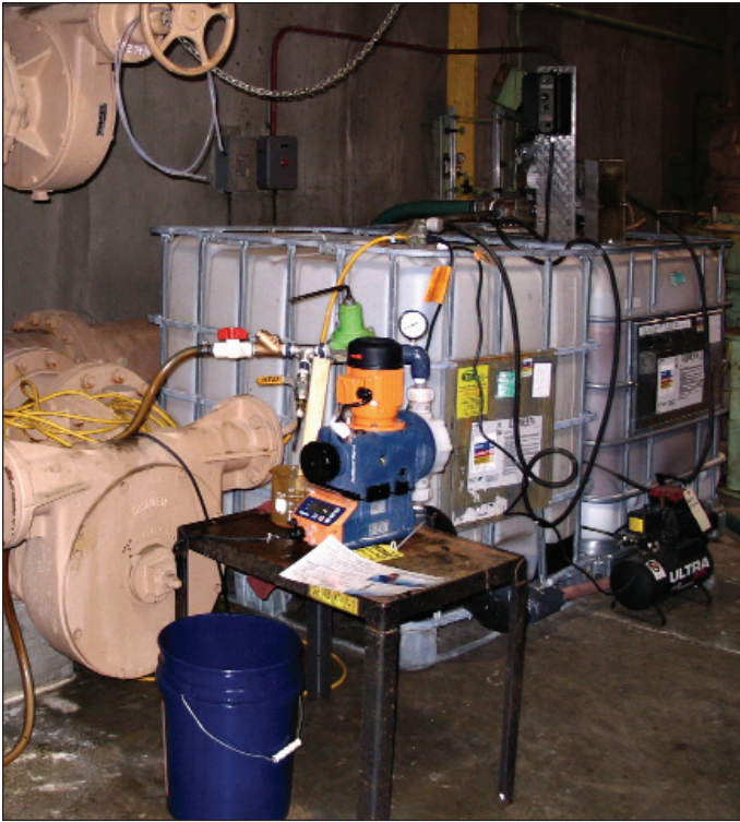
SDWRF carbon addition setup into mixing pump discharge.
